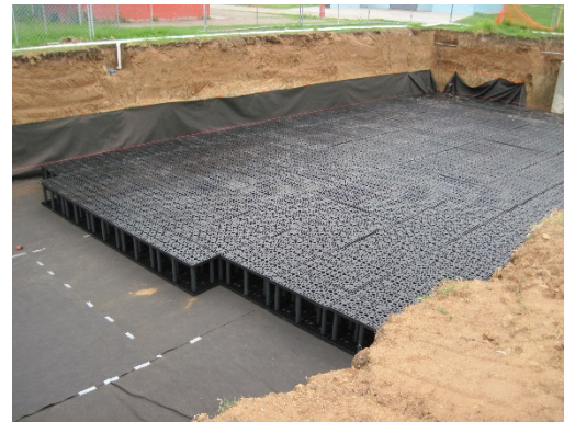
Figure 5-5. Subsurface infiltration gallery being constructed below a public park (source: Tetra Tech)
