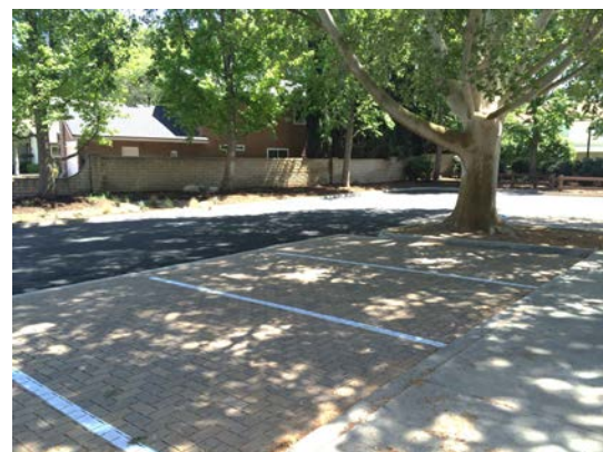
Figure 5-9. Permeable Paver Parking Lot - City of Santa Clarita Valencia Glen Park (source: City of Santa Clarita)
